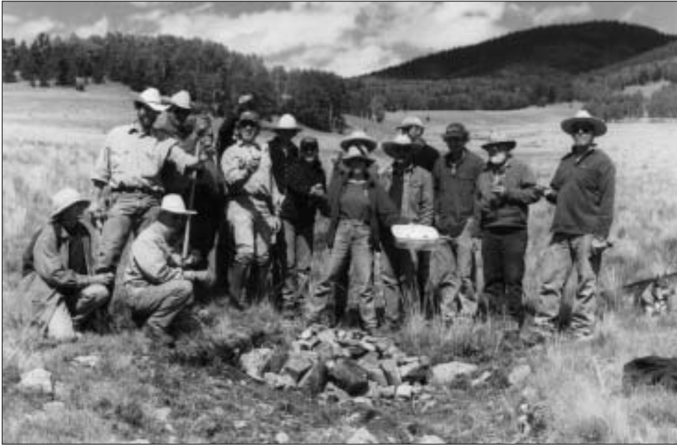
Volunteers “cupcake” toast to completed restoration work on a wet meadow in the Comanche Creek Watershed, Valle Vidal unit of the Carson National Forest, NM.
